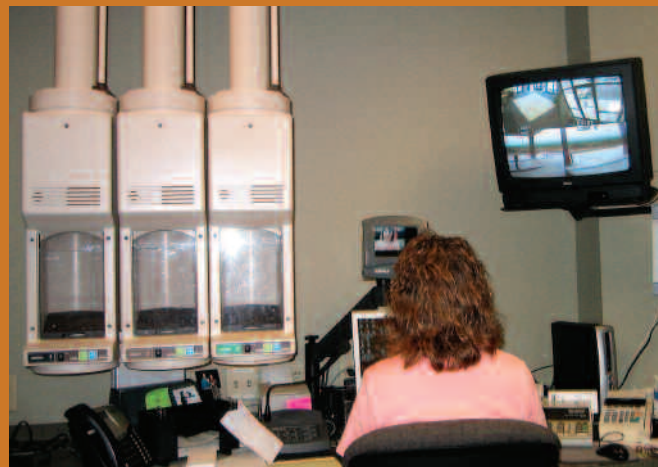
Remote Access —First American Bank and Trust's "remote teller" branch uses monitors, not windows for customer service touch-points.
